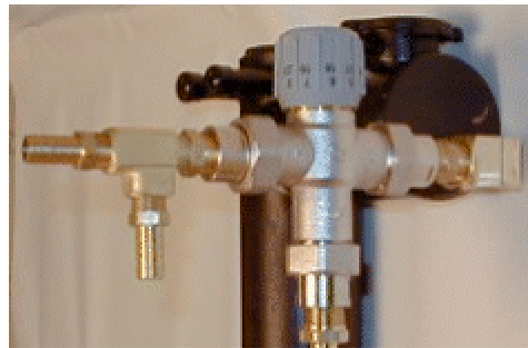
TCV mounted 90 degrees to female NPT fitting on Heat Exchanger
