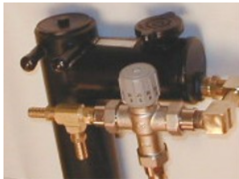
TCV mounted 180 degrees to female NPT fitting on Heat Exchanger
